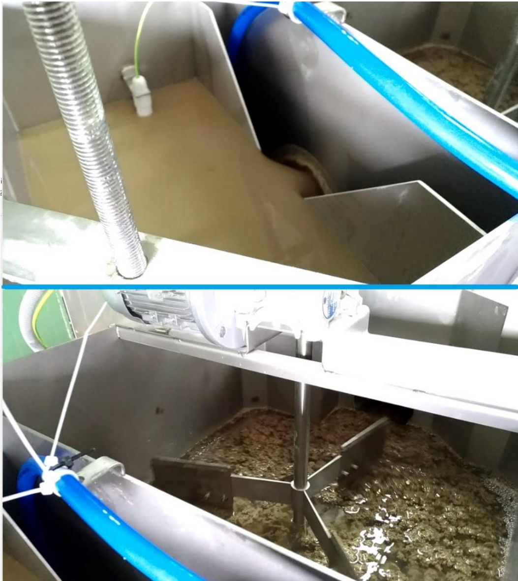
Fig. 12: Polymer effect – raw sludge in the inlet chamber without flocculant (upper) and optimal flocks in the mixing chamber (lower)
